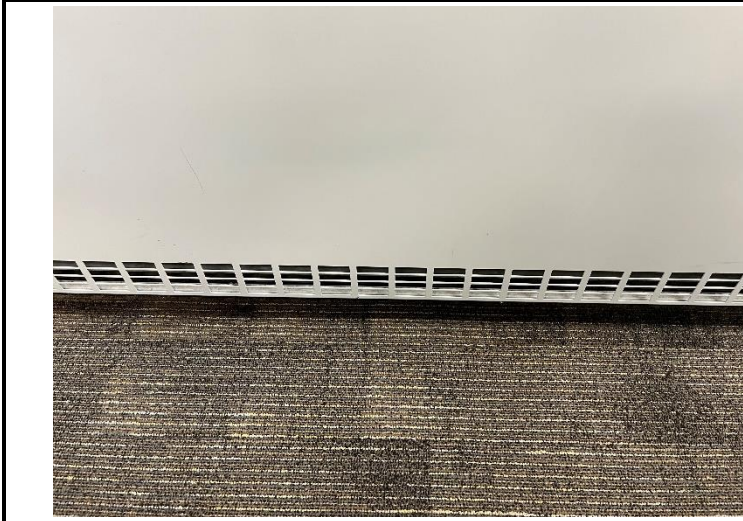
2. Stained carpet was observed in Room 120 near the unit ventilator.
