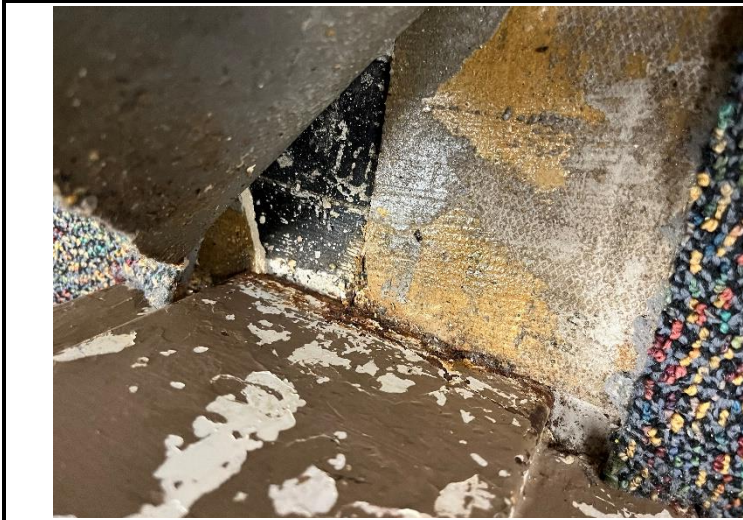
4. 9" x 9" assumed asbestos containing floor tile was observed under the carpet in Room 129.
