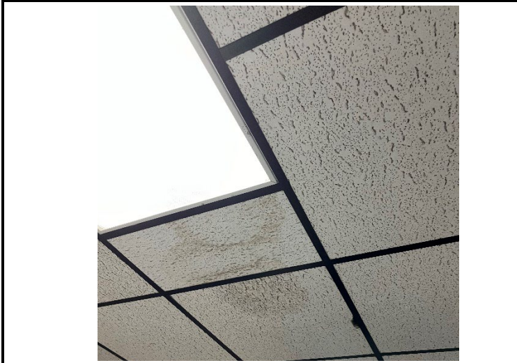
39. Water-stained ceiling tile was observed in Room 122.
