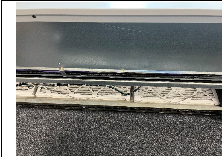
77. Merv filters were observed in the unit ventilators.
