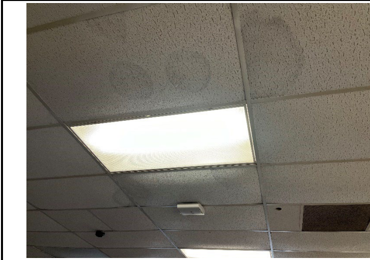
32. Room 127 had water-stained ceiling tile.
