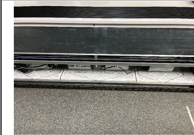
75. Inside unit ventilator in Room 107.
