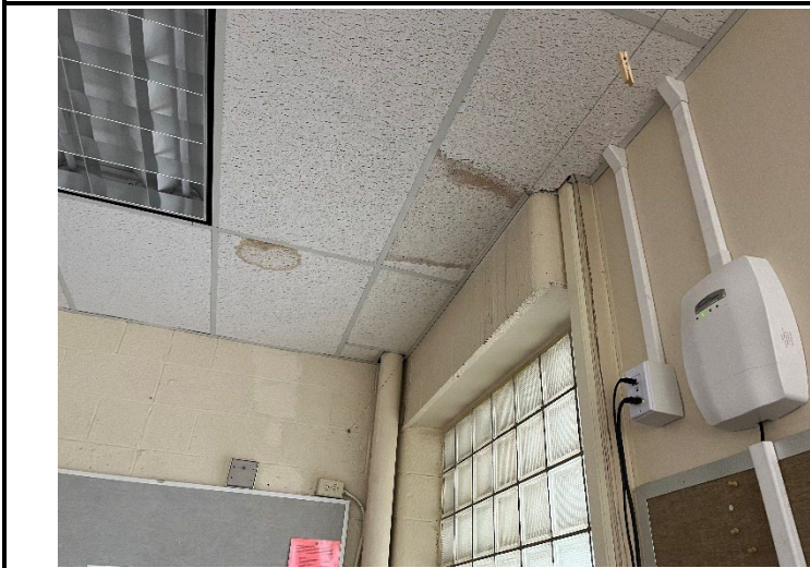
63. Room 105 water stains were observed on the wall.
