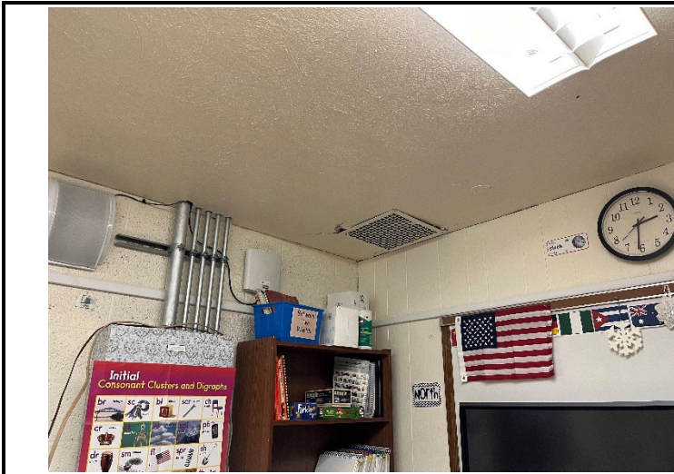
28. Room 125 had a damaged plaster ceiling.
