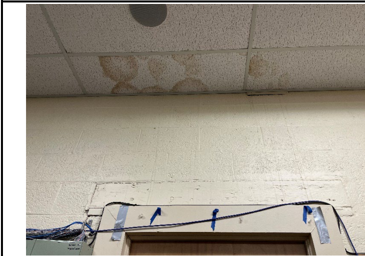
57. Water-stained ceiling tile was observed in the Library.
