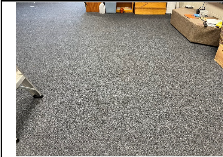
31. Stained carpet was observed in Room 129.
