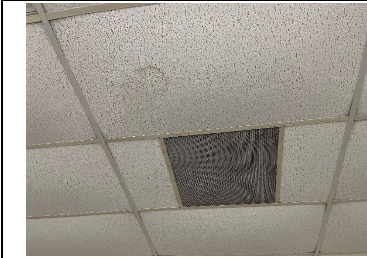
38. Water-stained ceiling tile were observed in Room 129.
