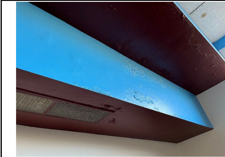
72. Bubbling paint was observed in the cafeteria.
