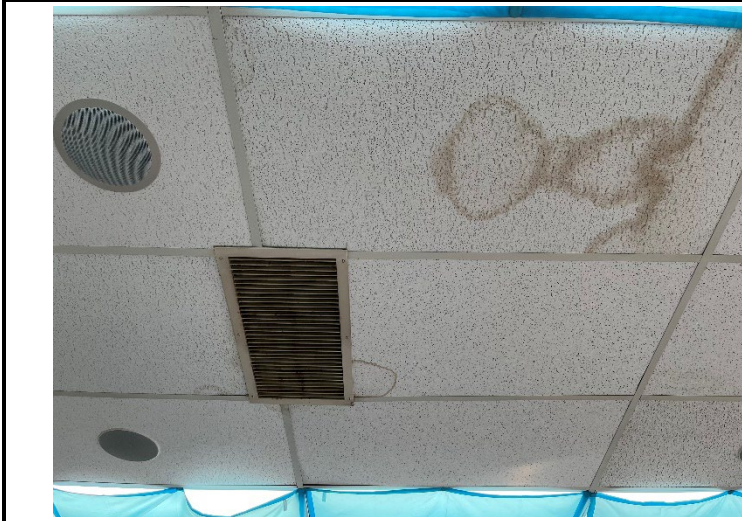
14. Water-stained ceiling tile were observed in Room 124B.
