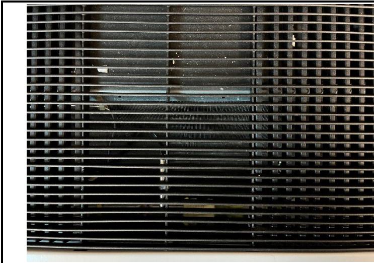
46. The unit ventilator was observed to be slightly dirty in Room 120.
