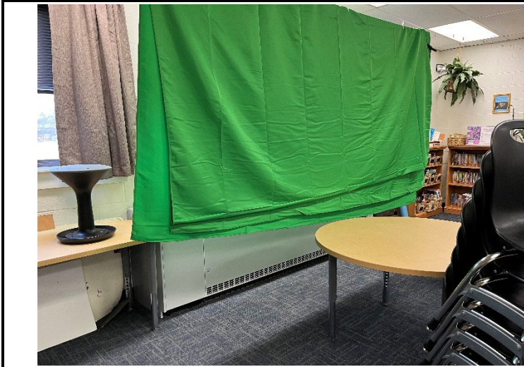
37. A cloth was observed to be in front of the unit ventilator in Room 129.
