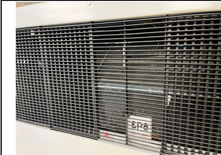
60. The unit ventilator was observed to be slightly dirty in Room 103.
