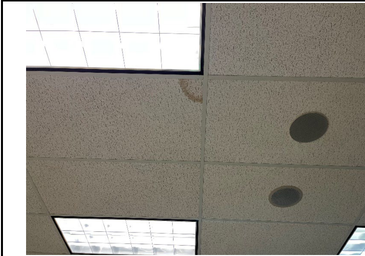
58. Water-stained ceiling tile was observed in the Library.
