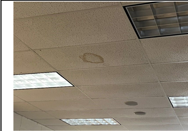
66. Water-stained ceiling tile was observed in Room 135.
