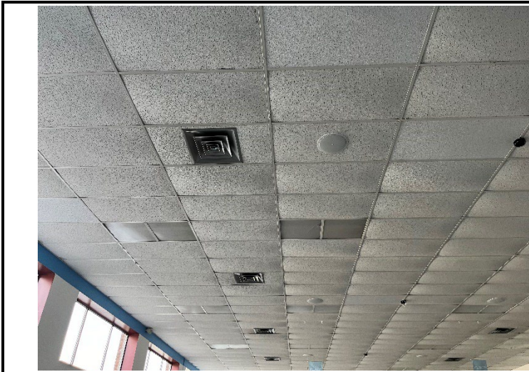
73. Bowed ceiling tile were observed in the cafeteria.
