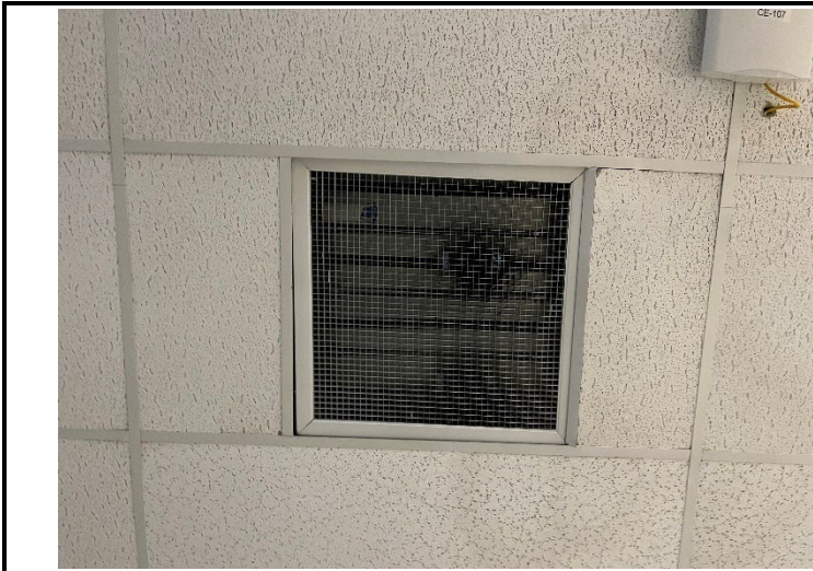
64. Dirty grille was observed in Room 107.
