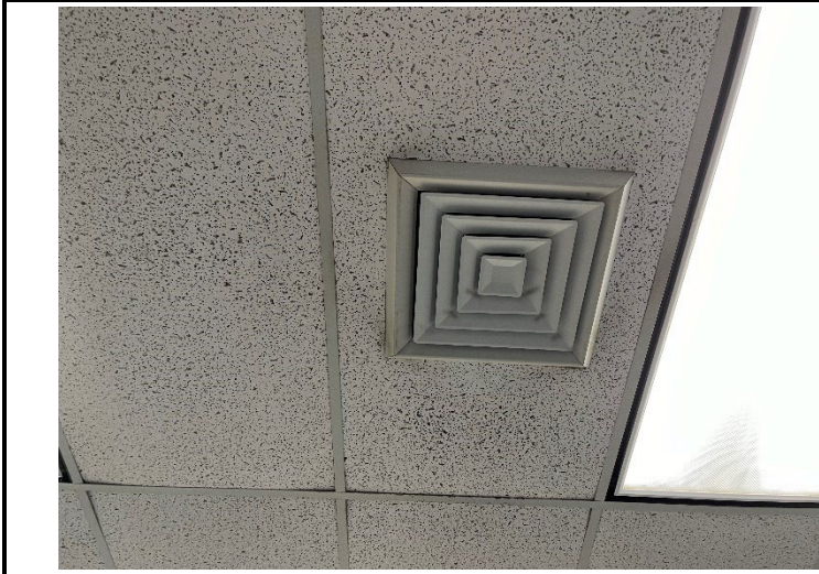
74. Soot-stained ceiling tile were observed in the cafeteria.
