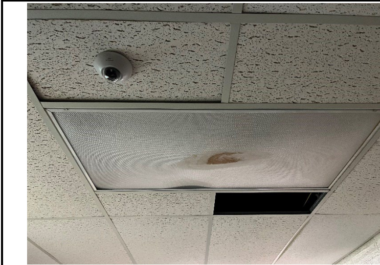
48. Water stains were observed in the light in the hallway near the Peace Room.
