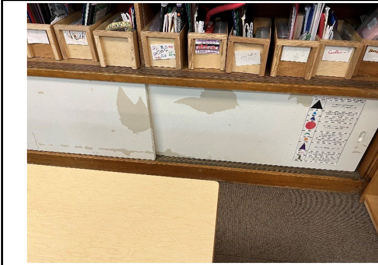
47. Peeling paint was observed on the cabinet in Room 120.
