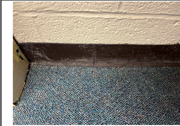
71. Room 110 white spots were observed on the cove molding.
