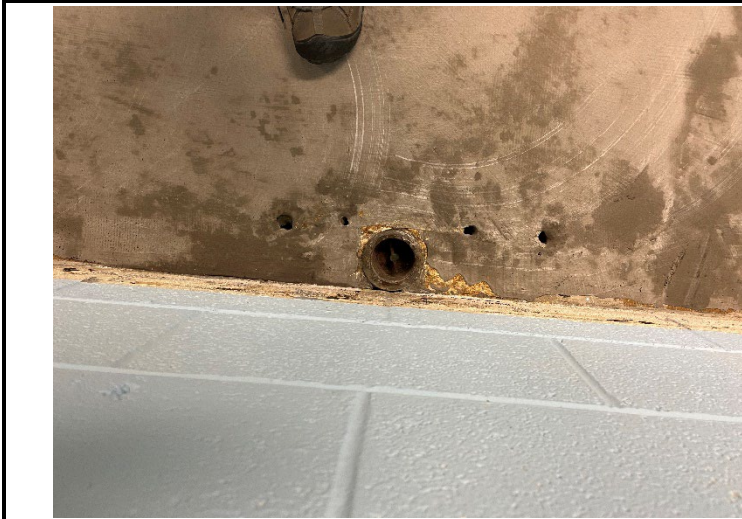
30. A capped drain was observed in the Peace Room 126. These openings were covered by a floor leveling compound installed as part of flooring replacement.
