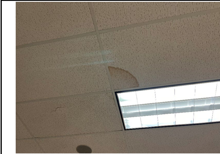
61. Water-stained ceiling tile was observed in Room 104.
