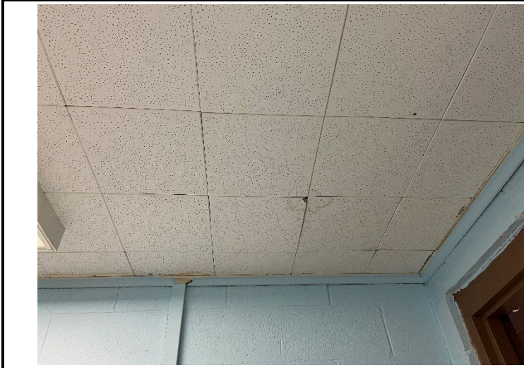
29. Water-stained ceiling tile was observed in Room 125.
