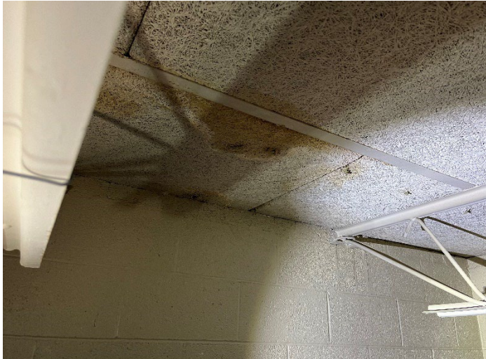
20. Mold was observed on the tectum decking above the drop ceiling tile in room behind 124B (124E).
