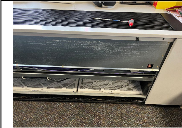
76. Room 107 inside the unit ventilator.
