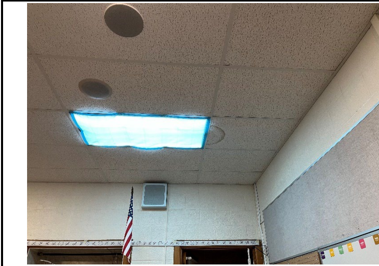
45. Water-stained ceiling tile was observed in Room 120.
