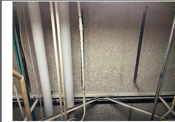
11. Water stains were observed on the ceiling in the Janitor's closet near the Gym.
